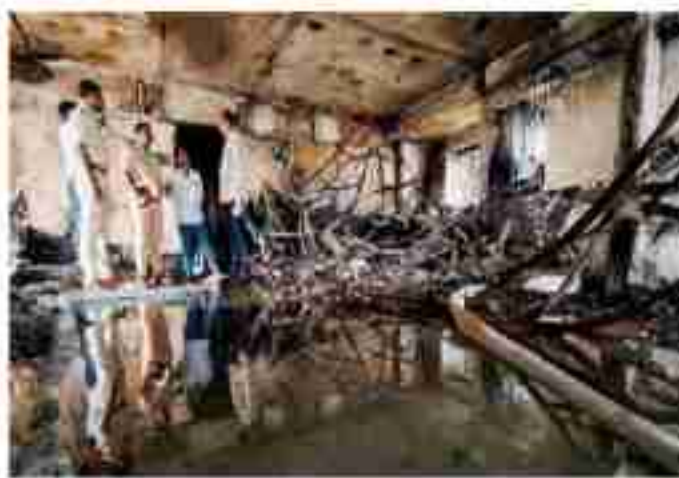
Charred walls: Police personnel conducting an inspection after a fire broke out at Rajeev Residency II MIM Complex, in Vashi, Navi Mumbai early on Tuesday (N).
