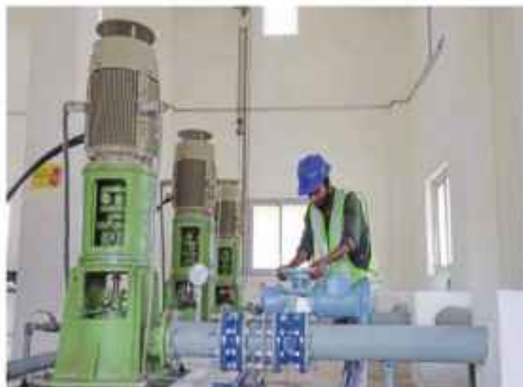
By focusing on capacity building and skill development, JM is ensuring efficient operation & maintenance of water supply systems
